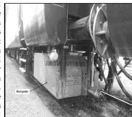
FIGURE 3: BIO TOILET INSTALLED IN A TRAIN
